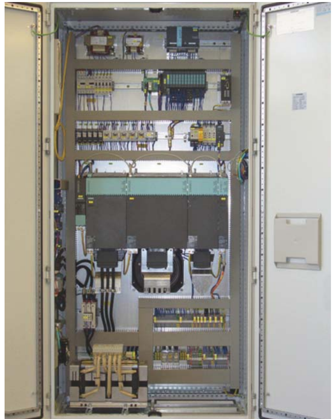
Control cabinet with SINAMICS
